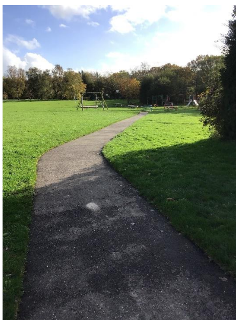
New path starting at Main Street and running to the play park on the Jubilee Field, Beckley
